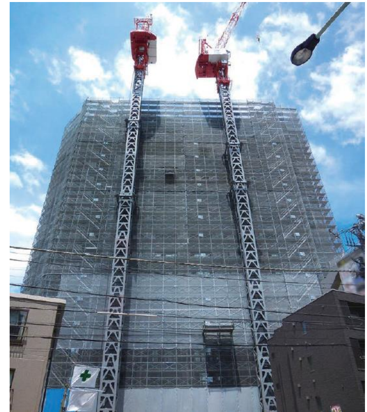
Scaffolding at this 80-meter condominium project begins at the B2 level and has a total height of 90 meters
